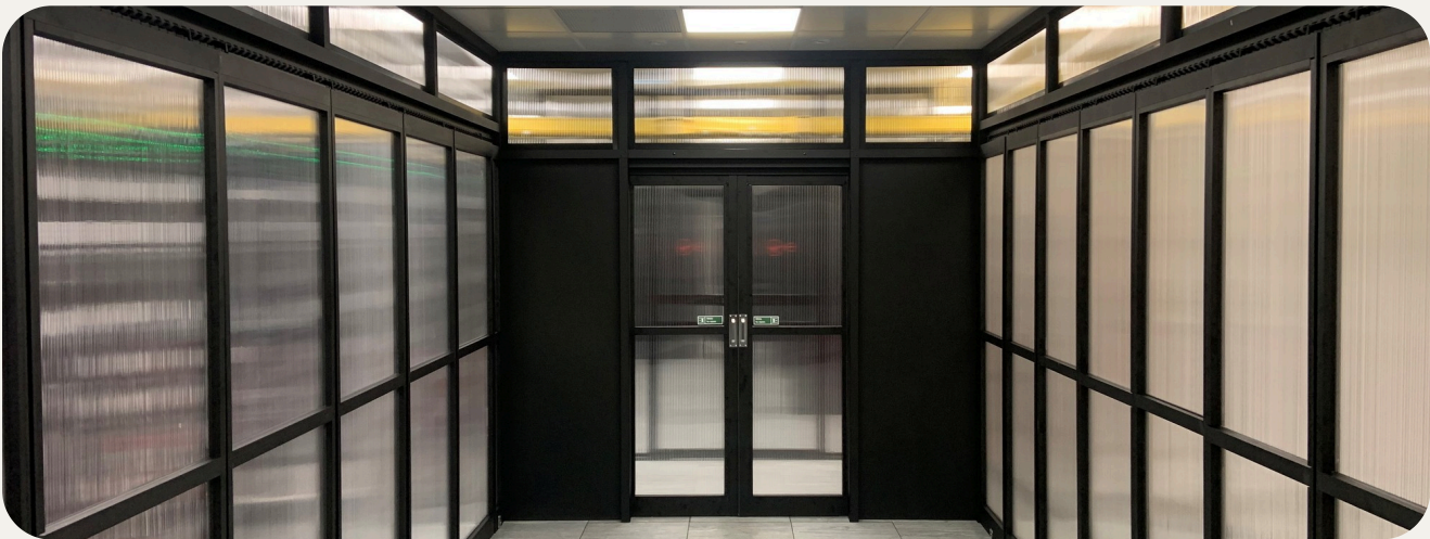
Installed FastFix enclosure, Northampton. View the project online →
